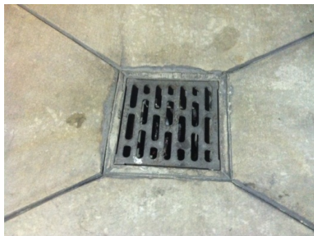
Rear Ramp Drains
