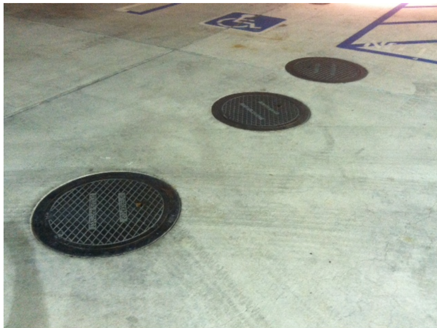
Clarifier lids at station 105
